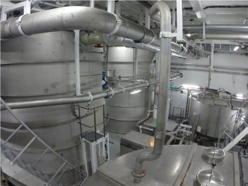
Scanship wastewater treatment system on RCCL Quantum of the Seas
